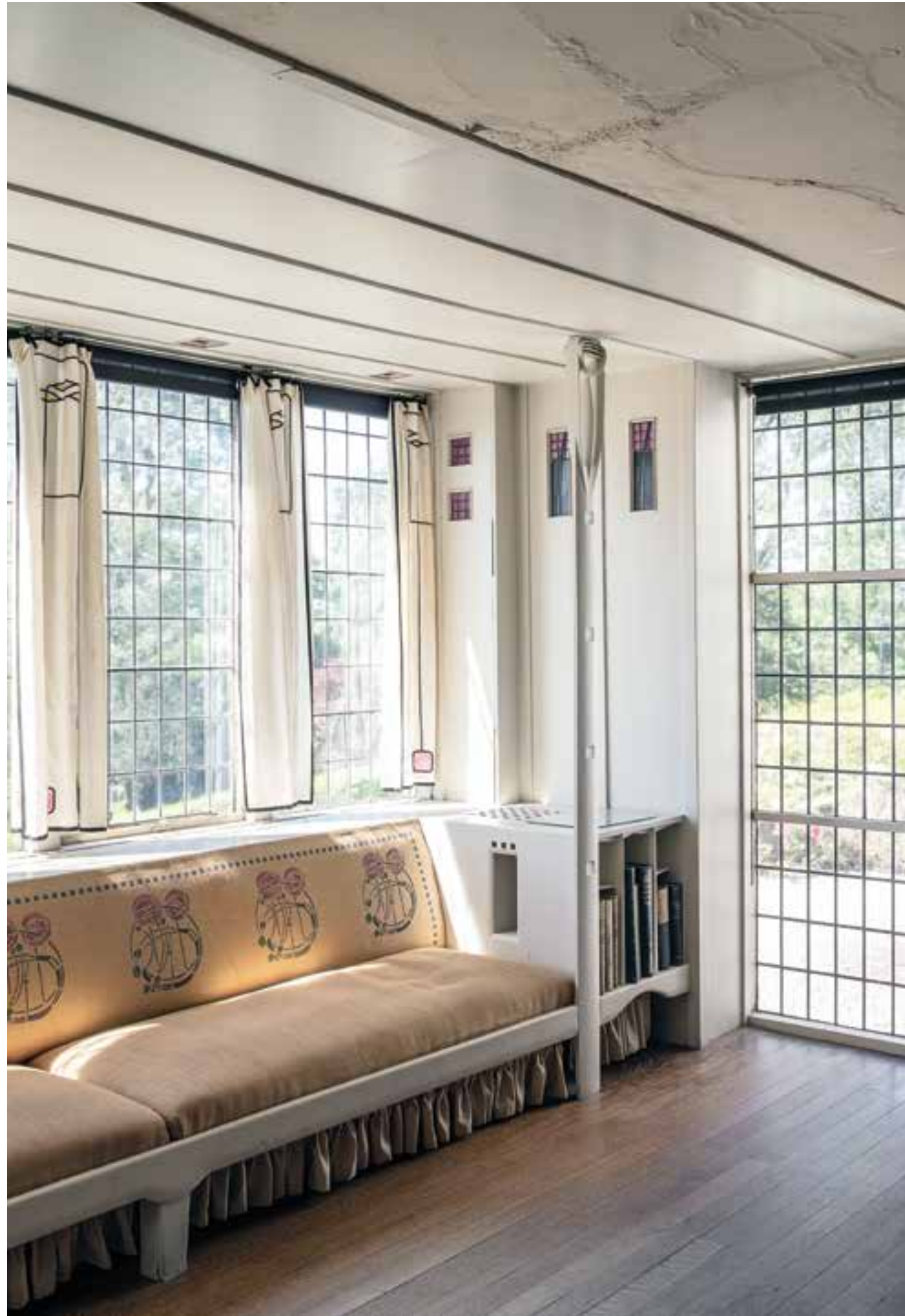
SHADOWS AND LIGHT Left: Overlooking the garden, a heated window settee in the white drawing room has stenciled-burlap upholstery—and extensive water damage overhead. Opposite: Level changes and a switchback staircase lend the dimly lit entry hall a sense of spatial dislocation.
